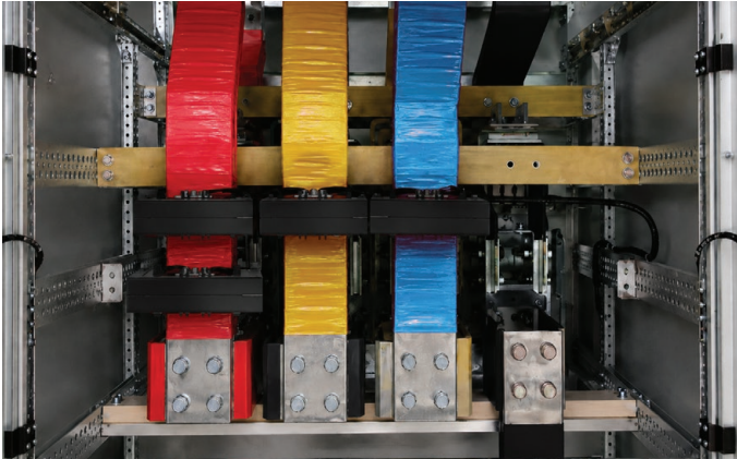
Figure 1: Installation of AcuCT-3147A on Insulated MV Bus Conductors in Switchgear Panel
